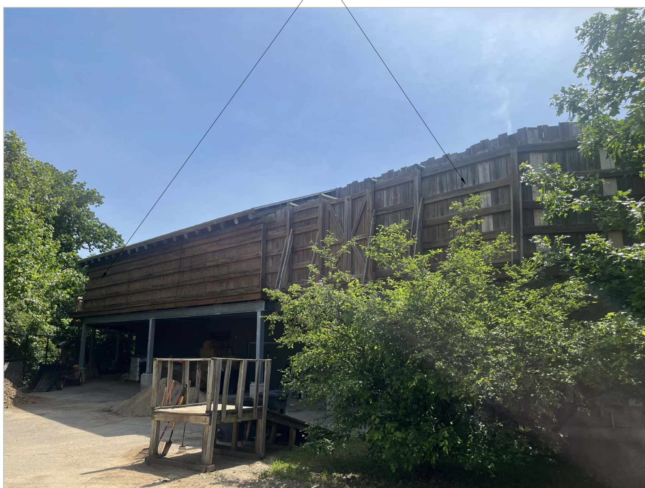
4 Fence Photo at Staff side of Rhino / Giraffe Nighouse A2 NO SCALE
