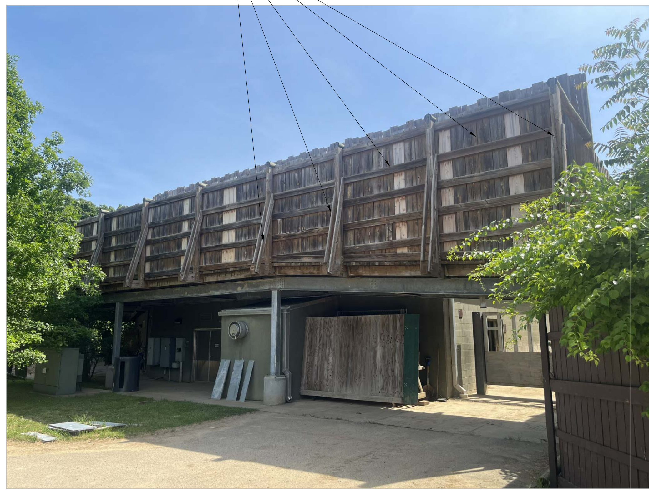
1 Fence Photo at Staff side of Rhino / Giraffe Nighouse A2 NO SCALE
